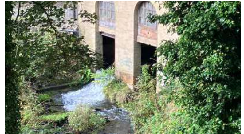
Images of Ovenden Brook and culverts (near the site - Brook not accessible on site)
